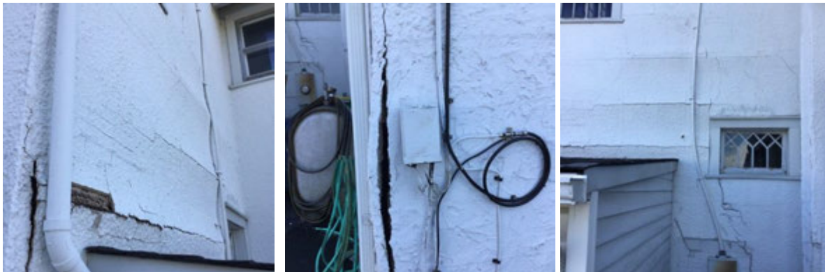
Images of exterior deteriorating
