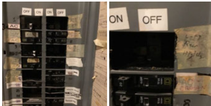
Images of open breaker spaces
