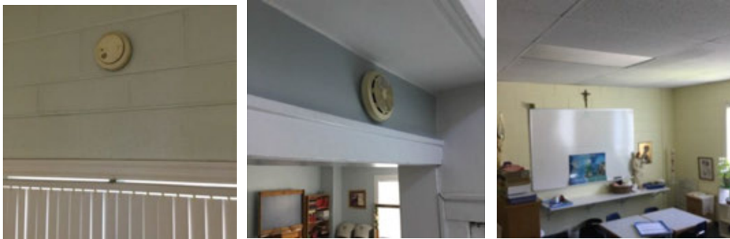
Images of outdated and missing smoke detectors
