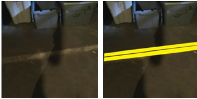
Images of uneven concrete
