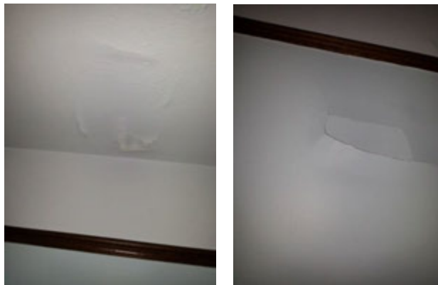
Images of paint cracking
