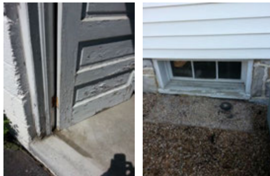
Images of paint peeling
