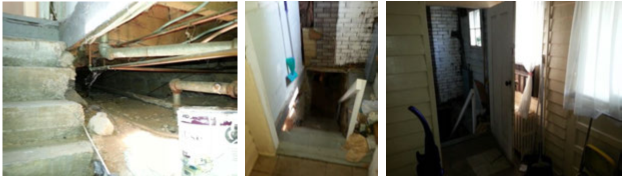
Images of open fire breach and basement entrance
