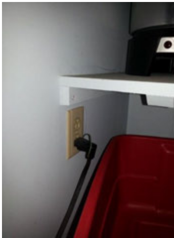
Image of improper wiring
