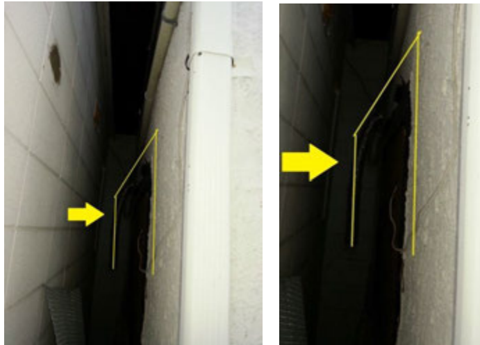
Images of hole in wall
