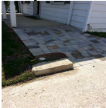
Images of trip hazard
