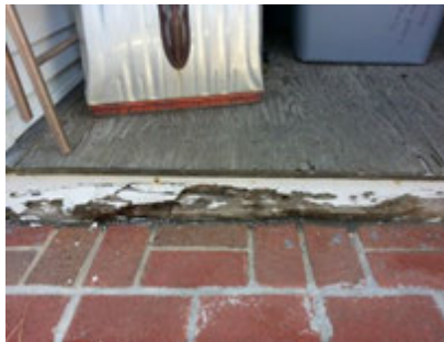
Image of evidence of water damage and un painted exterior
