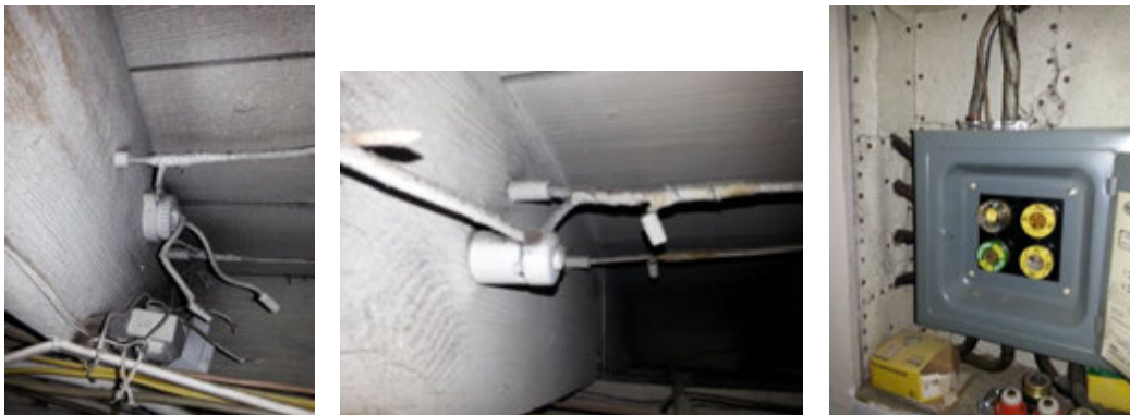
Images of knob and tube wiring still in service and other outdated wiring
